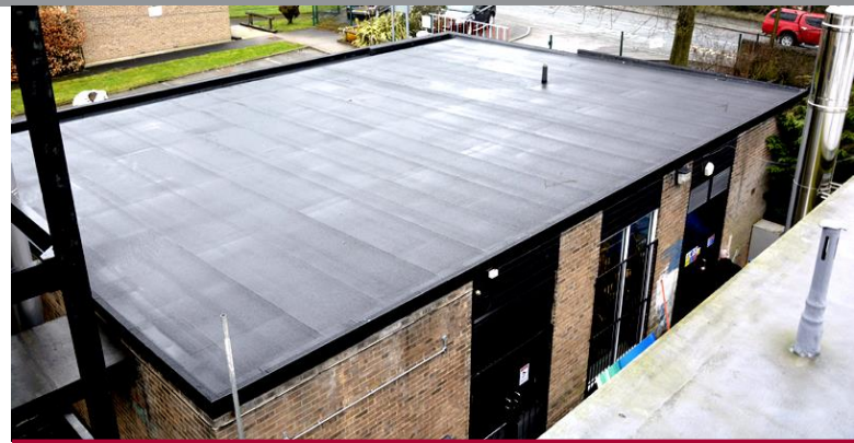
Stripping the roof away on the boiler house revealed a rusting metal deck due to water sitting in the deck troughs
