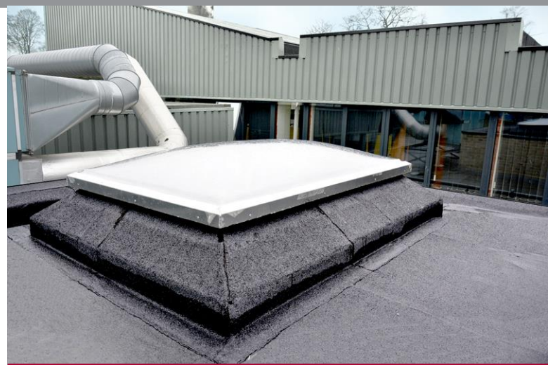
The existing fragile glass roof lights have been replaced with triple skinned roof domes which have been tested for safety and strength
